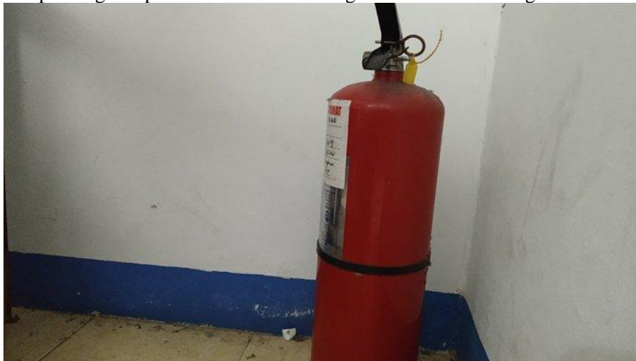
Figure 9. Availability of Fire Extinguisher (APAR)
