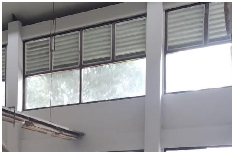
Figure 2. Air Ventilation in Workshop
